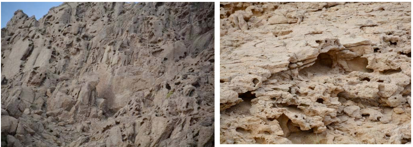
Honeycomb weathering in Dammam and limestone
